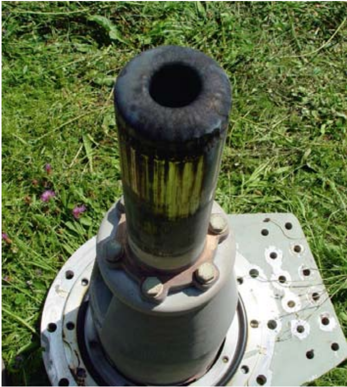
Fixed inner contact of a high-voltage circuit breaker. The erosion can clearly be observed (photo: Weis)
